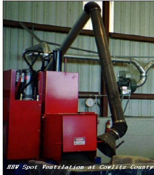
Local Ventilation connected to Hepa Filter
